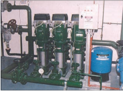
Hydrovar variable-speed drives
