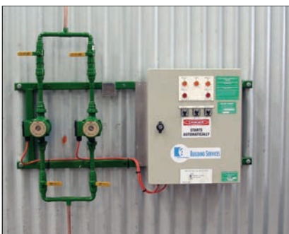
Packaged system hot water circulator
